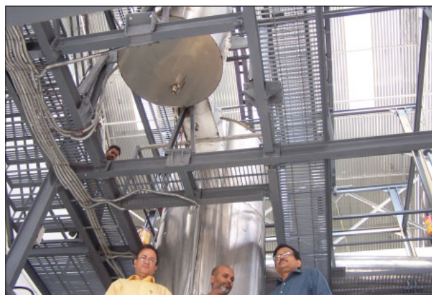
The reactor which converts plastics waste into fuel
